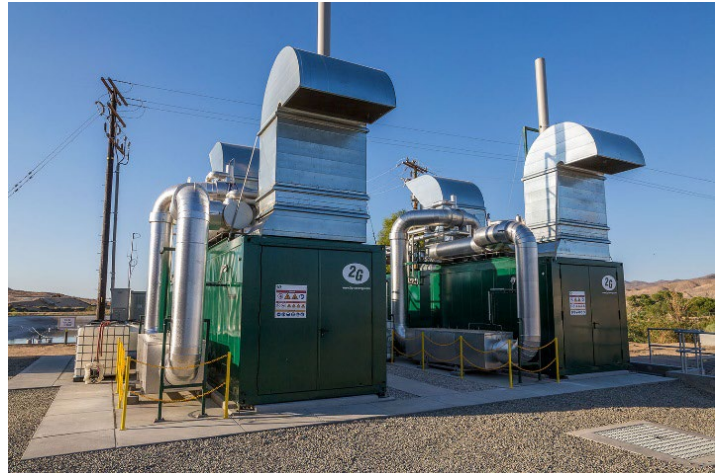
Figure 6: Anaergia’s 1.6 MW e Biogas CHP at the Victor Valley Wastewater Reclamation Authority in Victorville, CA
