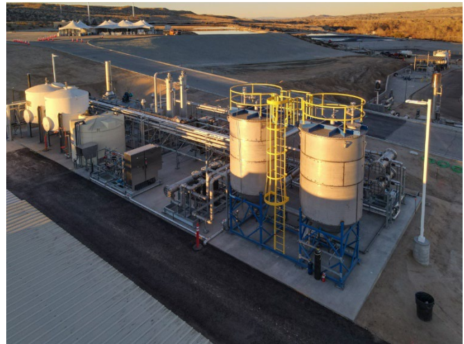
Figure 5: BUG at a California WWTP
