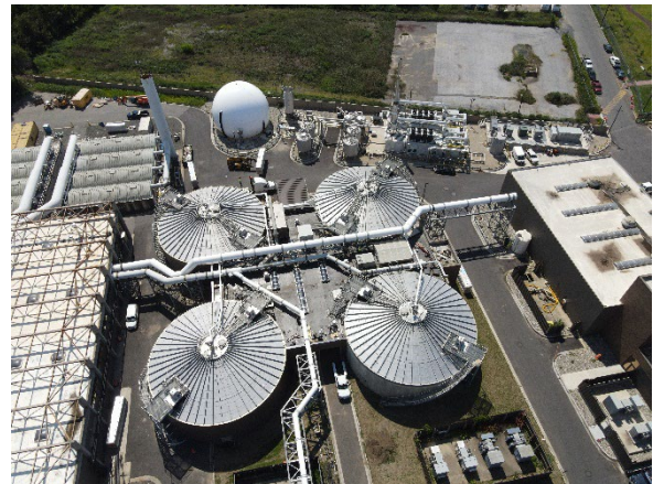
Figure 4: Camden County WWTP AD and Co-Generation Facility
