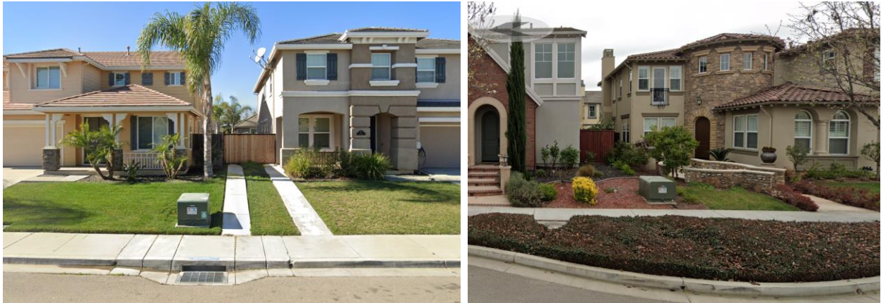
Figure 1: Examples of Pad-Mounted Transformer Installations
